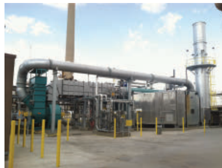
200,000 lb/hr package watertube boiler with CataStak™ SCR system and EconoStak economizer, designed and supplied by Nationwide Boiler Inc.
