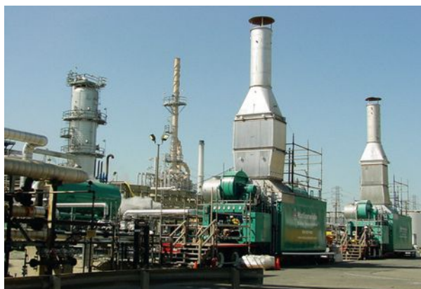
RENTAL BOILERS SIMILAR TO THESE 70,000 LB/HR UNITS WITH CATASTAK™ SCR SYSTEMS MUST BE CONSIDERED DURING THE PLANNING PROCESS OF A COAL TO NATURAL GAS-FIRED CONVERSION PROJECT.
