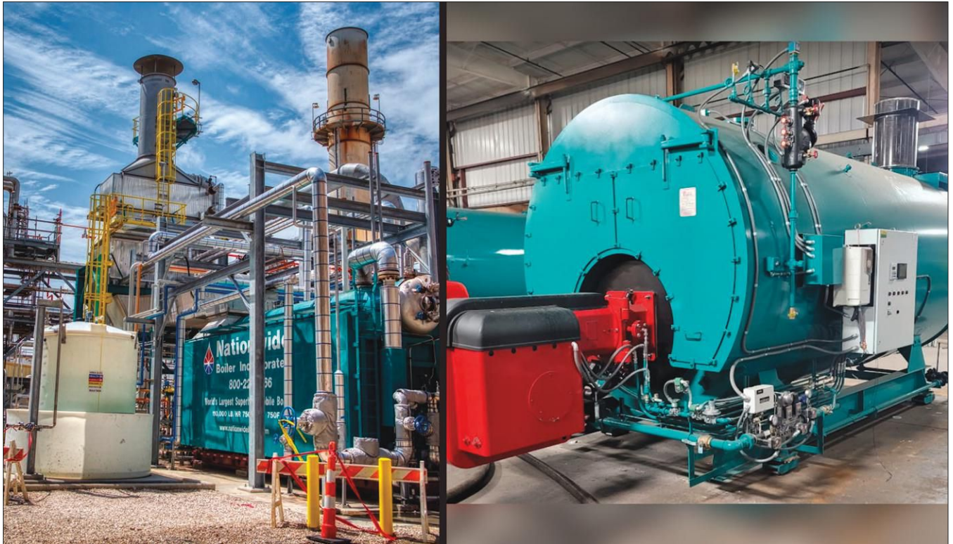
FIGURE 1. A 110,000-pound-per-hour package watertube rental boiler and CataStak™ SCR for single-digit NO x compliance (left) and a 350-hp package firetube boiler with proven 2 ½ ppm ultra-low NO x burner (right). Image courtesy of Nationwide Boiler
