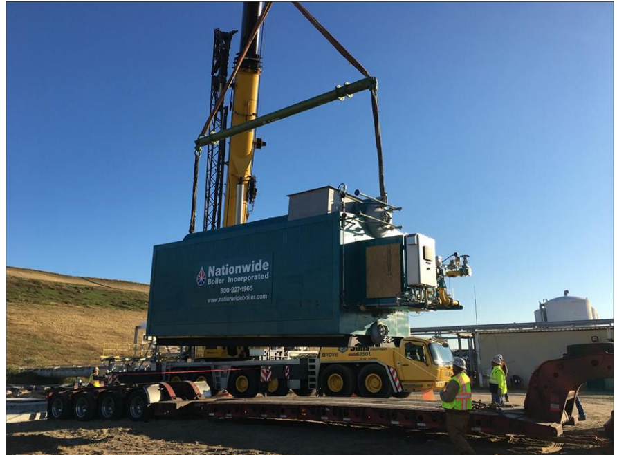
FIGURE 1. A 120,000-pound-per-hour DFW boiler sale that was completed last year. The boiler shown here was lifted off the trailer to be set in place upon delivery.
